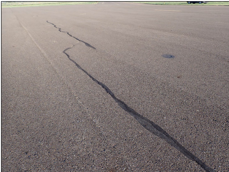
AP-15-12: L&T Cracking
