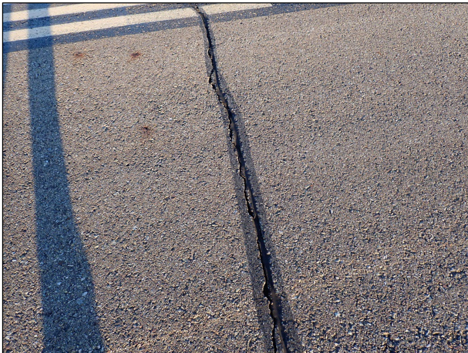
TW-13-03: L&T Cracking
